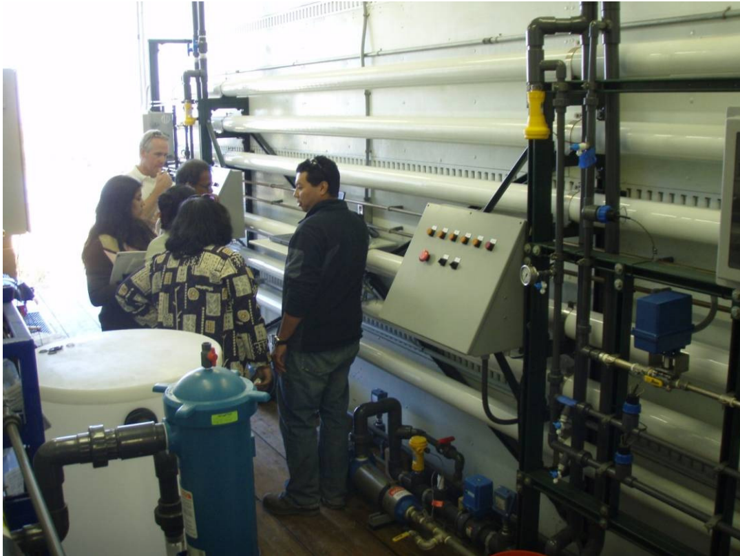
Figure 3-9: Photograph of RO Trailer
