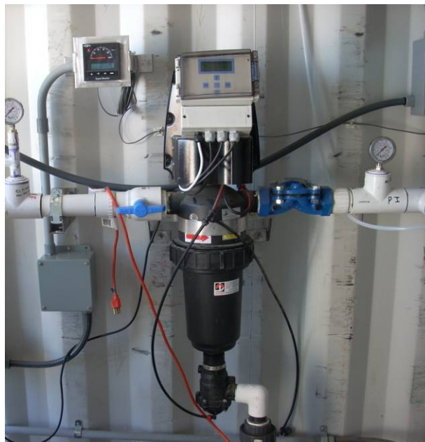
Figure 3-4: Amiad Self Cleaning Screen
