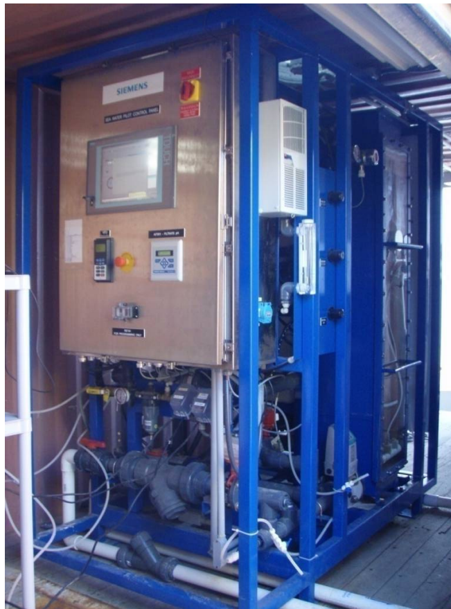
Figure 3-5: Submerged UF System
