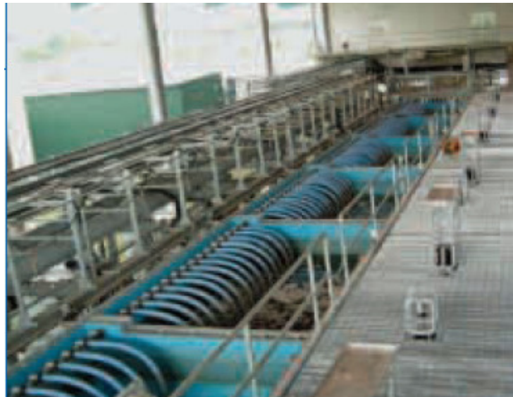
Figure 4-4. Siemens/Memcor Submerged UF Membranes
