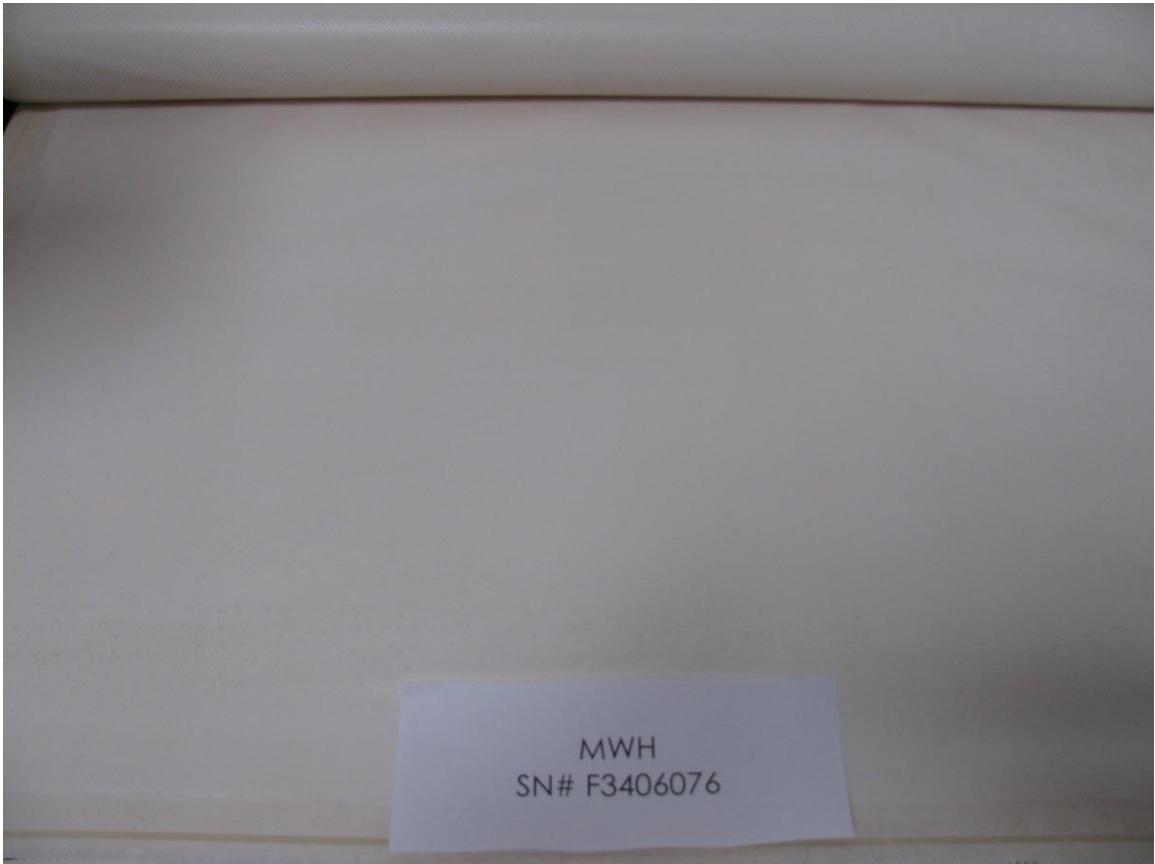
Figure 1: Exposed membrane surface for SN# F3406076.
