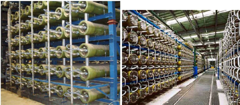
Figure 4-11 Typical Desalination RO Arrays
